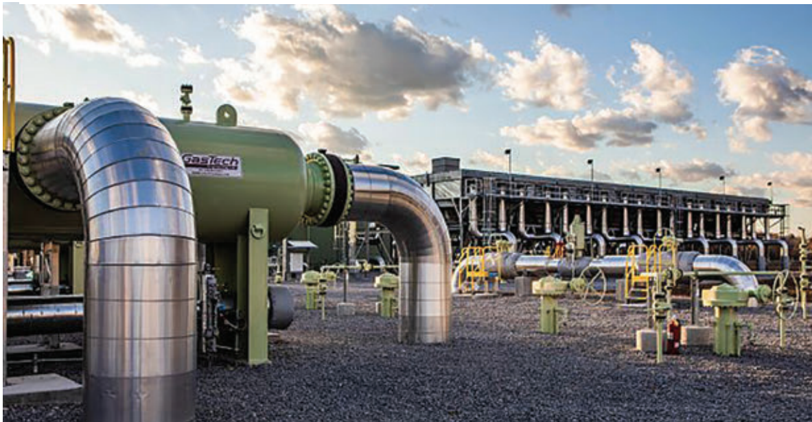
Gas transmission compressor station. (Source: TC Energy)
