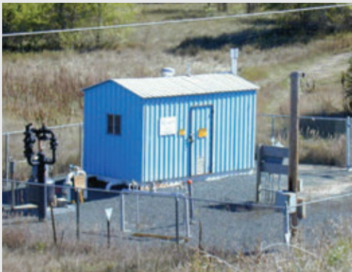
City gate meter station.
