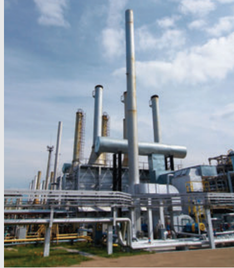
Natural gas processing facility.
