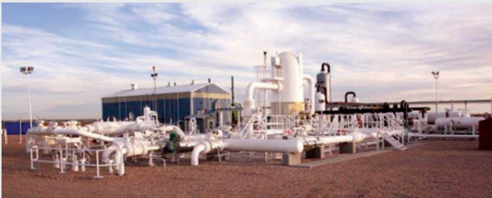
Natural gas compressor station.
